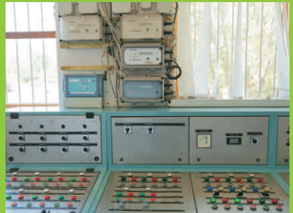
The control panel at Gansvlei
